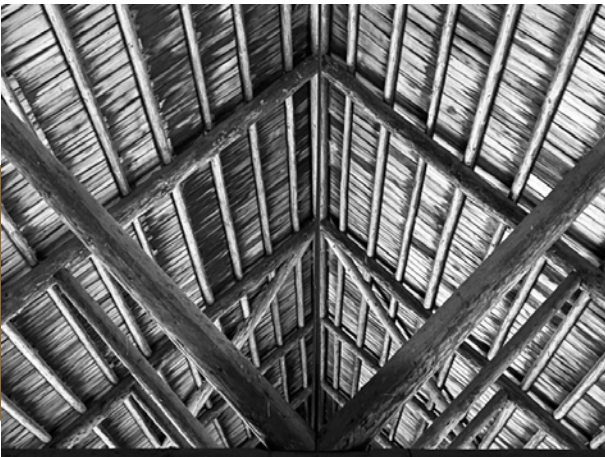
A spectacular view of the interwoven beams (scissor and ridge), struts, under purlins, props, and shingles.
